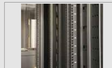
Front (rear) sides of cabinet with vertical PDU and wire trimmers
